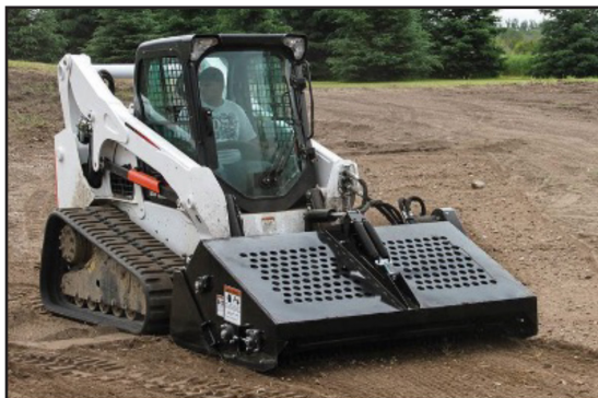
Example of skid steer with "Rockhound" (landscape rake) attached which is used in grading land.
